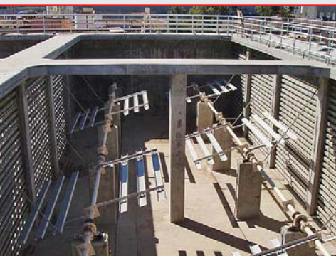
JMS Horizontal Flocculators
